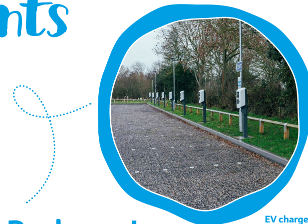
EV chargers in Lakeside car park
